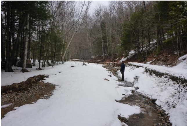
Figure 7 - Road washout area. The channel bed is almost as high as the floodplain in this section. The channel has aggraded and the river goes overbank during lower than normal flood levels. The river cut down thru the road bed about 4.5 ft. in depth for several hundred feet.
