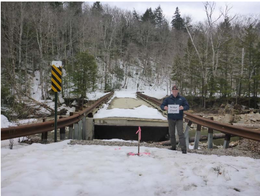
Figure 8 - Rocky Branch Bridge near road approach. Both abutment approaches were washed out and the abutment structure sustained damage to the concrete backwalls.
