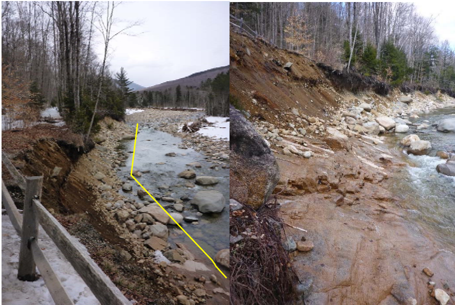
Figure 2 View looking upstream along the river bank adjacent to the trail/road. Note the fine grained materials and lack of large boulders along the toe of the bank. Yellow line designates the toe of the proposed riprap revetment
