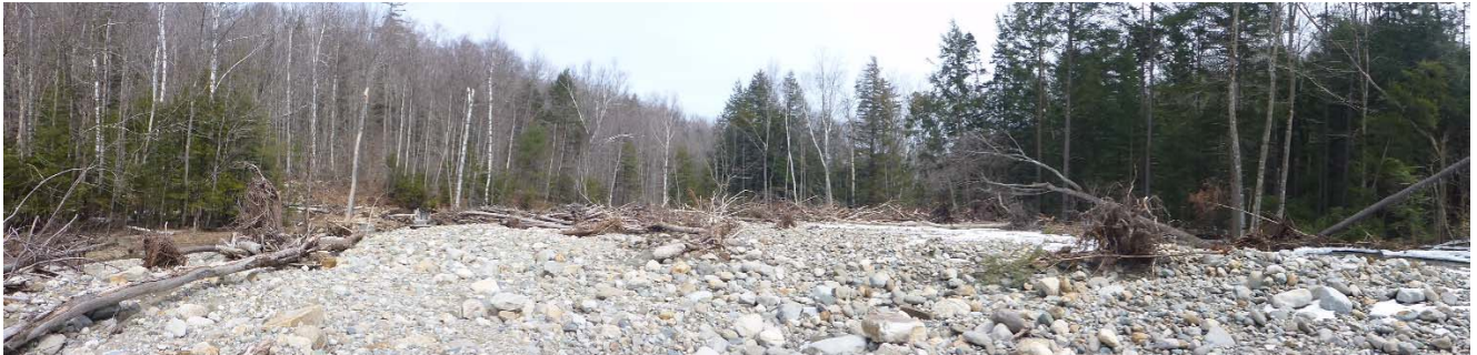
Figure 14 - Large alluvial fan has formed immediately upstream of the Town Bridge on Tunnel Brook. Sediment has built up 6 to 8ft in places and numerous cross valley log jams have formed helping to retain sediment on the alluvial fan.
